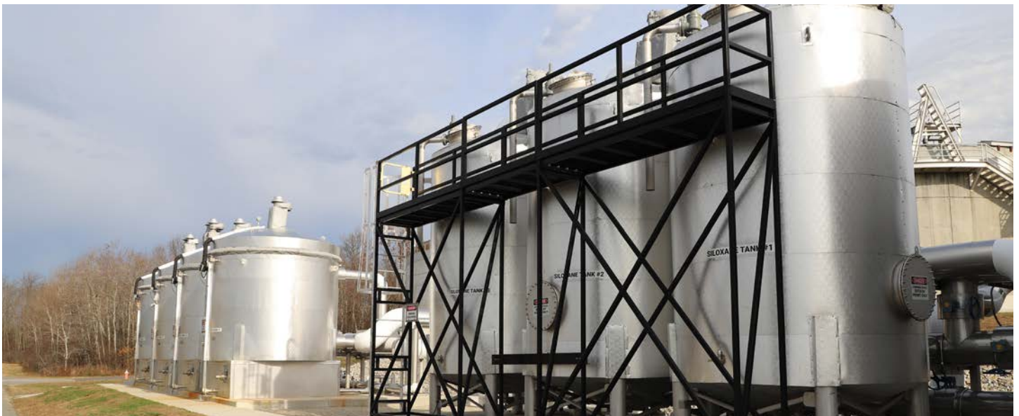
Organics to Energy Digester Facility, North Andover, MA
